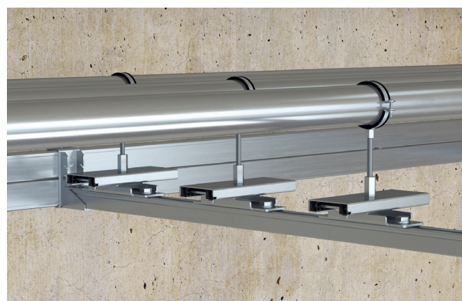
Hot water and circulation pipes
