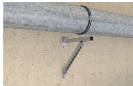
Spiral airduct on cantilever
