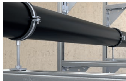
Connection on channel
