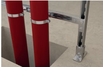
Waste water pipe
