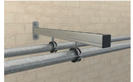
Pipelines on cantilevers
