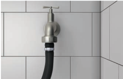
Outlet valve with hose
