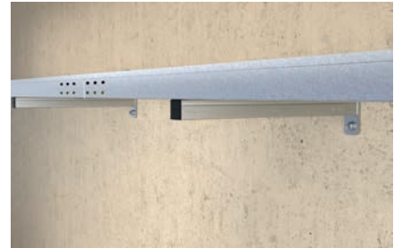
Cable tray on cantilever arm
